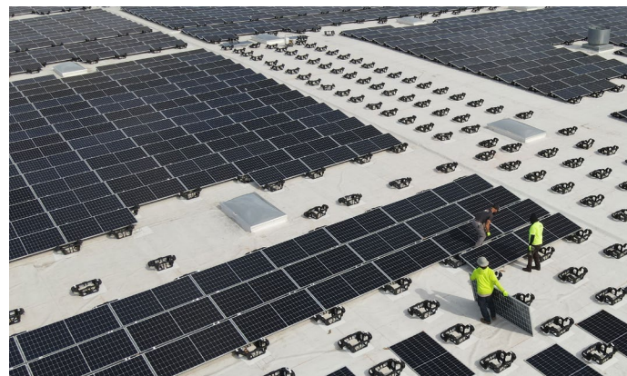
Solar array roof installation at an Avantor facility in California. Photo Credit: Redaptive
